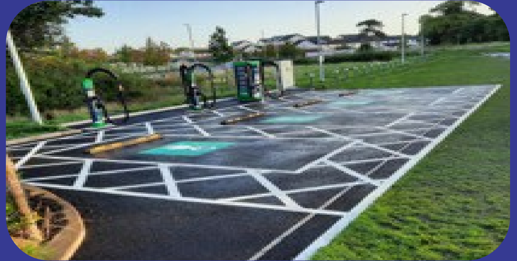
Public EV Charging at Tandy's Lane Park
