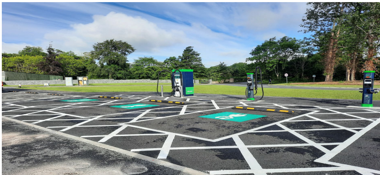
Newly installed fully accessible public EV charging in Corkagh Park
