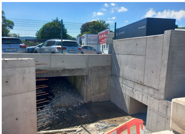
Flood defence walls at Whitechurch
