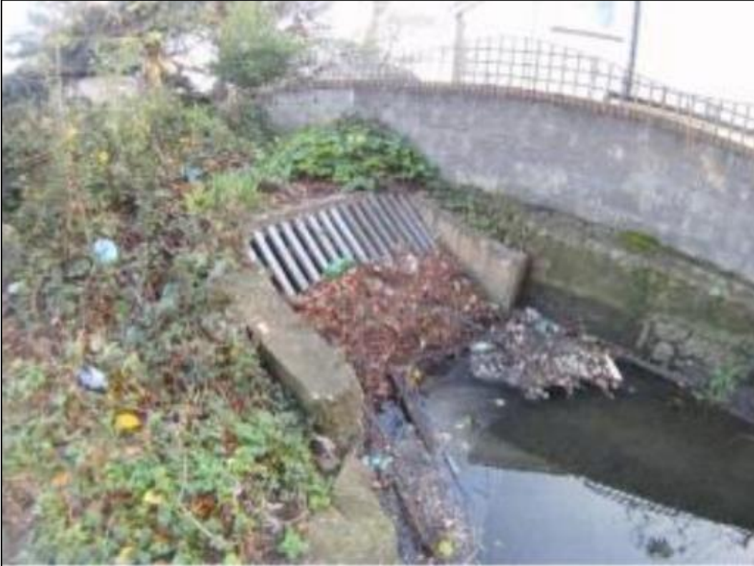
Figure 3-2: Blocked trash screen at Ballycullen culvert causing flooding in 2011 (Flood ID-11686)
