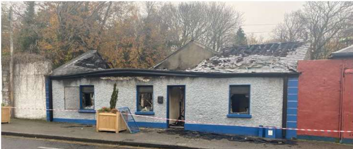
Figure 5 St Dominics Hall, still a derelict building after more than three years,
