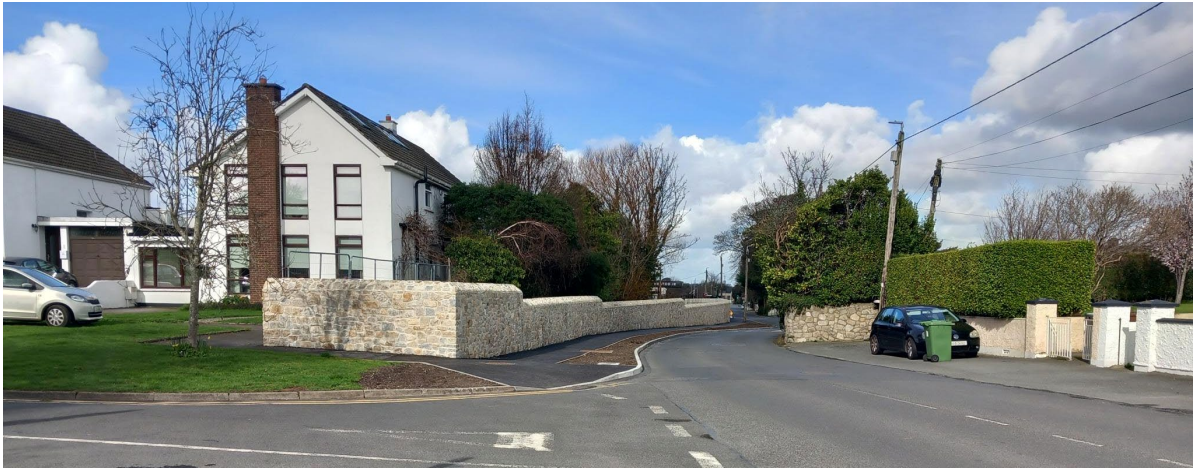
Completed flood defence wall at Whitechurch Stream (St. Gatien's Court-St. Enda's Drive)
