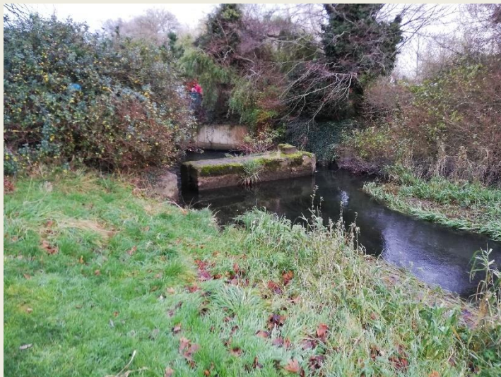
4) Looking DS: Redundant mill infrastructure remains in the channel, causing a barrier to flow and sediment transport.
