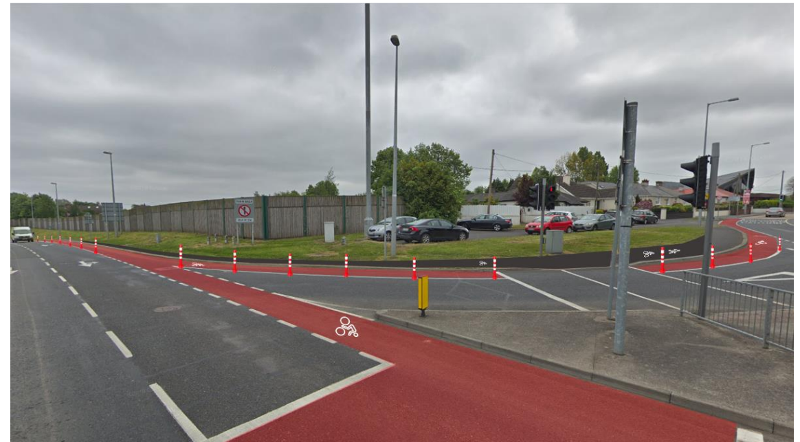
View of Leg 1 with new bollards, cycle track and restoration of red surfacing.
