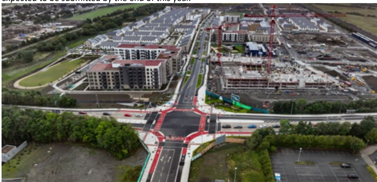
Eastern section of Southern Link Street in Clonburris SDZ and adjoining residential development
