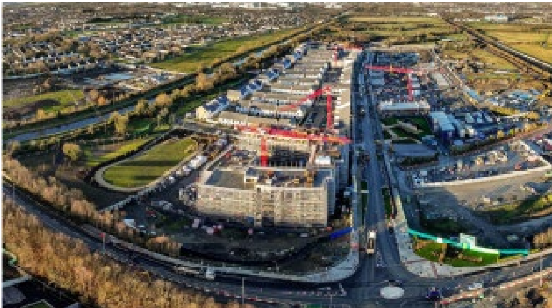
Eastern section of Southern Link Street in Clonburris SDZ and adjoining private residential development
