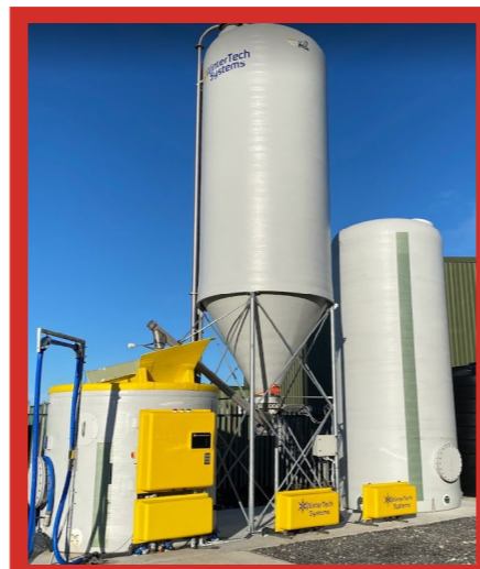
Brine Saturation Facility
