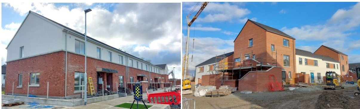
Work is progressing on the significant social housing developments at New Nangor Road(L) and Balgaddy (R)
