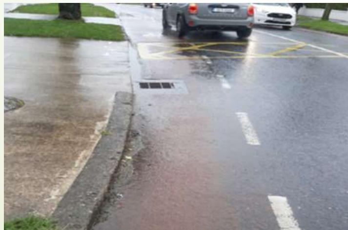
Level 3 - No surface defects but poor appearance (cycle track markings could require refreshing)
