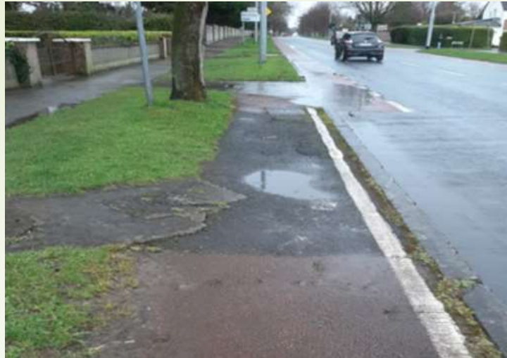
Level 1 - Major surface deterioration (loss of wearing course, potholes and structural defect, & tree root uplift)
