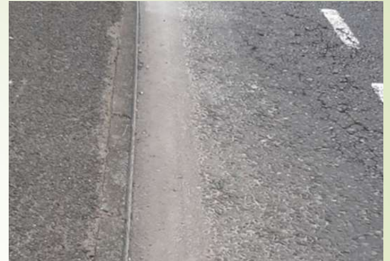
Level 2 - Minor surface defects (surface cracking, ravelling)
