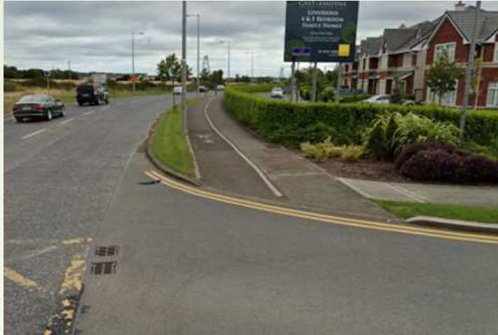
Level 1 - Cyclists give way to side road traffic with no crossing features provided for them. May be unclear who has right of way.
