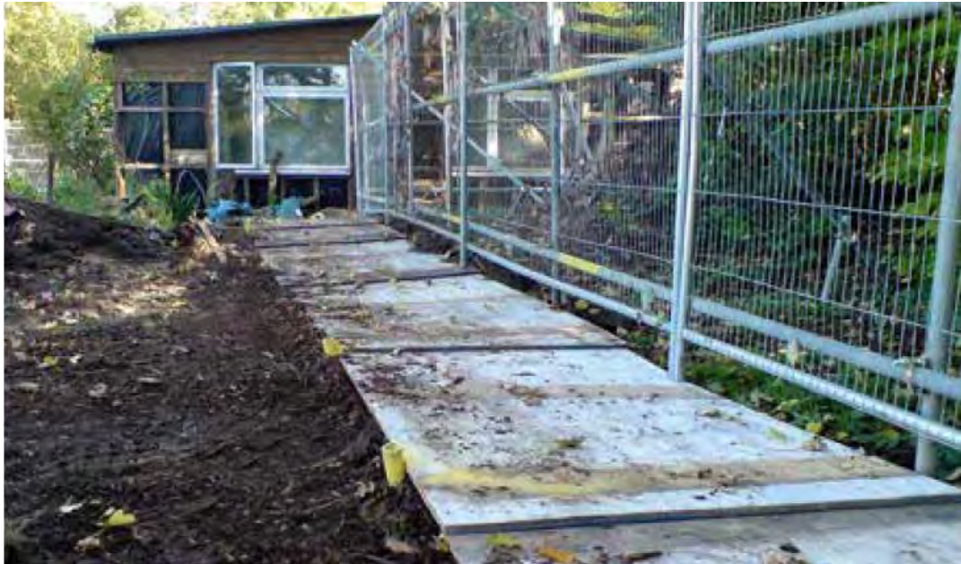
Figure 2: An example of temporary ground protection. The 150 mm woodchip is spread on top of a geotextile membrane and heavy-duty plywood is pinned in place to spread the loading and prevent compaction of the underlying soil.
