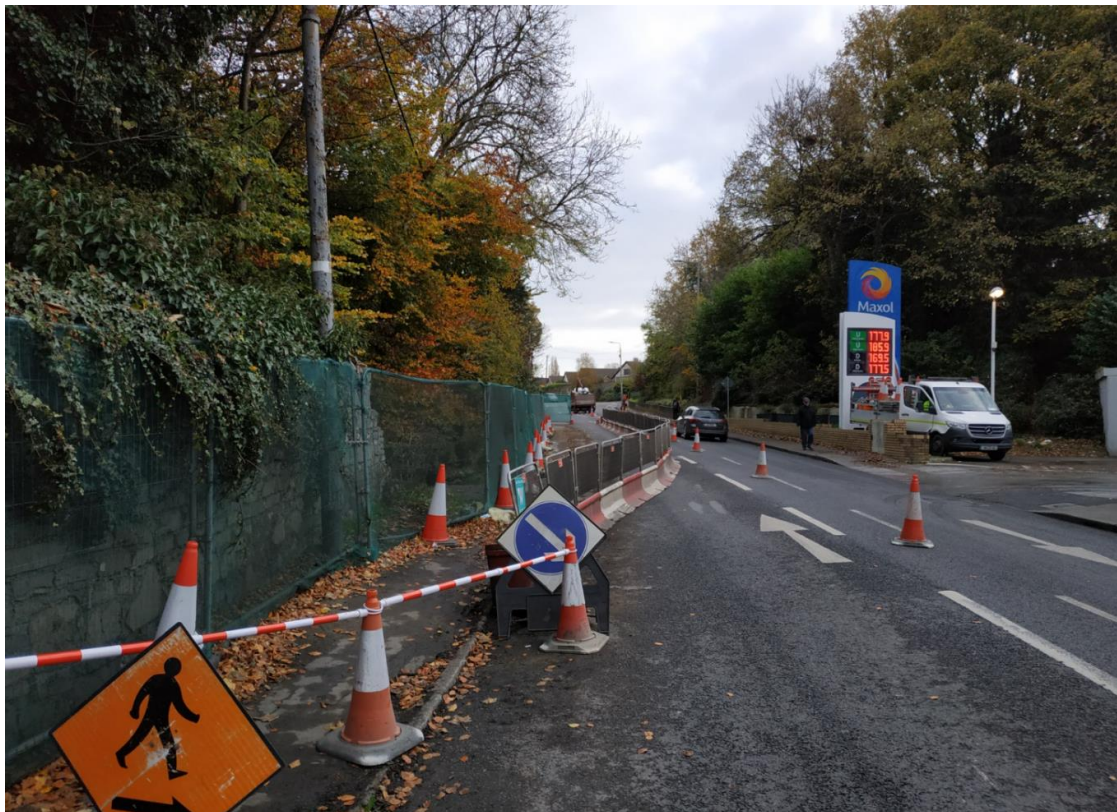
Photograph 1 Looking to the East. R835 Road with Traffic Management System in place during the ground investigations. Retaining Wall at the left side
