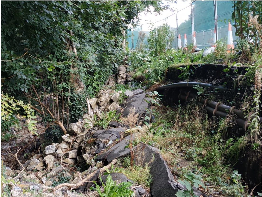
Photograph 6 Collapsed retaining wall section. Services exposed
