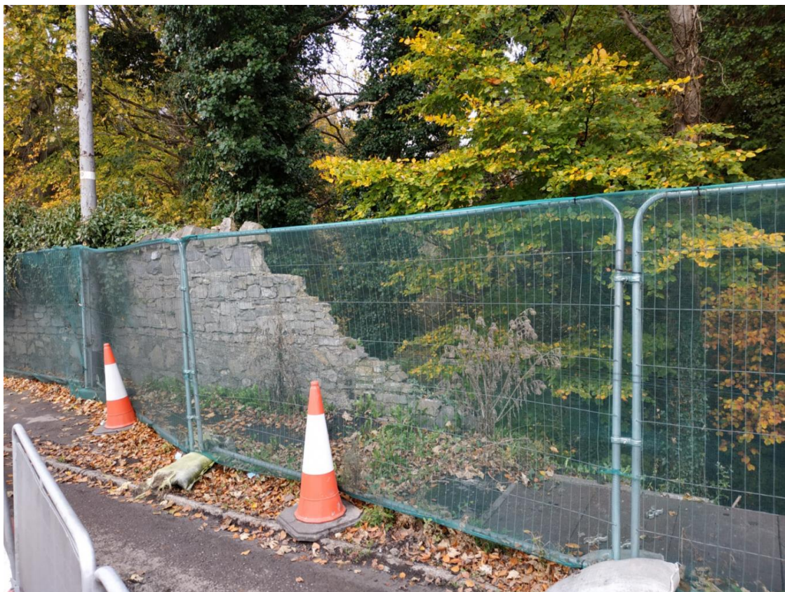
Photograph 3 Retaining wall failure
