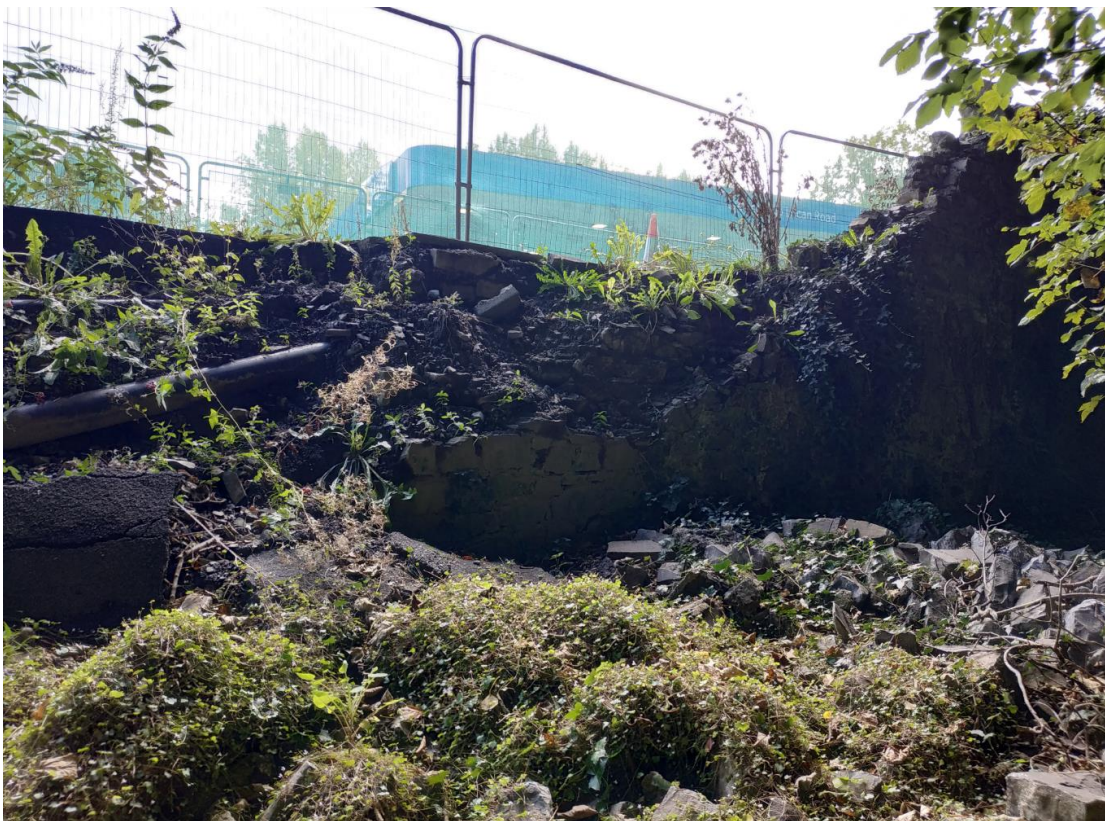
Photograph 7 Collapsed retaining wall section. Services exposed
