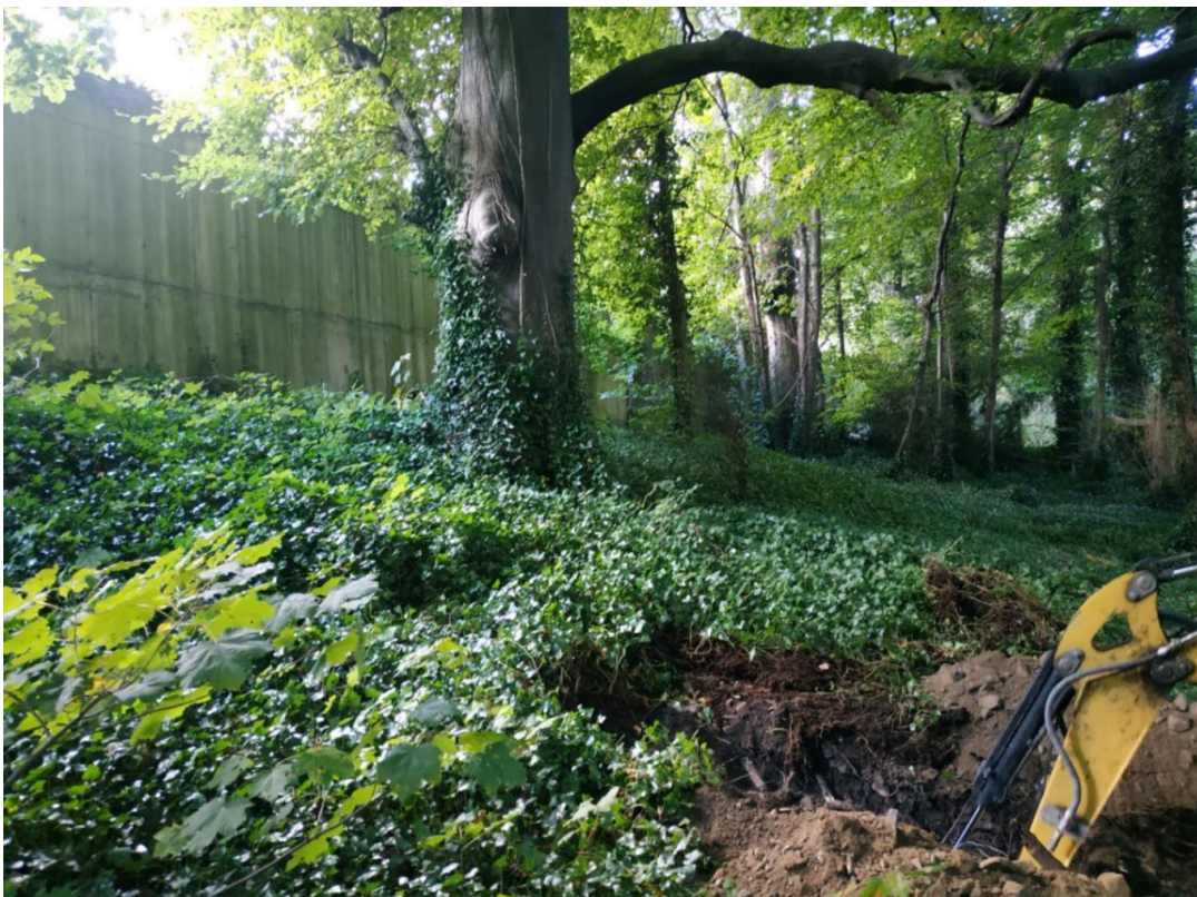
Photograph 9 Looking to the West. The ground slopes down to the North towards River Liffey (image taken during ground investigations)
