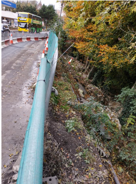
Photograph 2 Looking to the West. View showing the location of the collapsed wall which is the boundary between the green land area and the R835 Road retained by the wall before its failure
