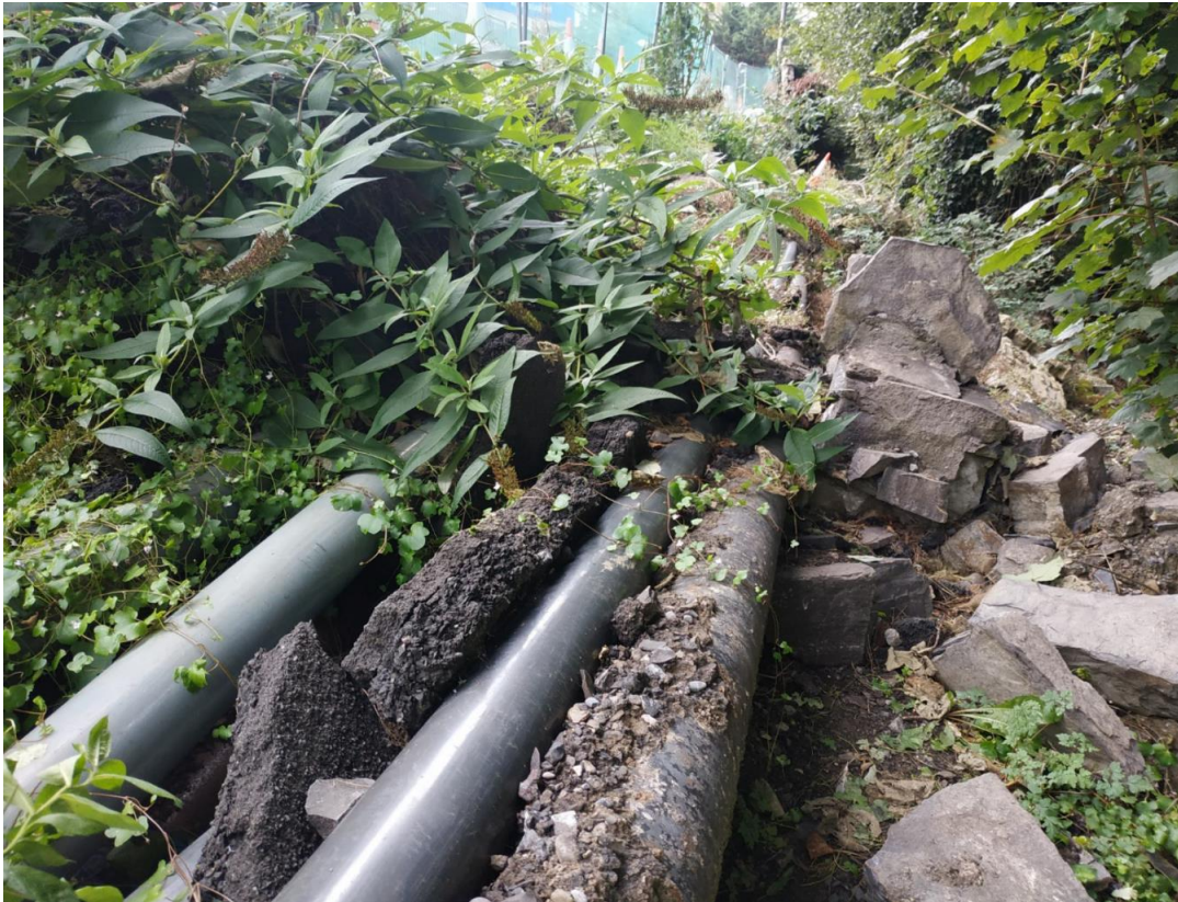
Photograph 8 Services exposed following collapse
