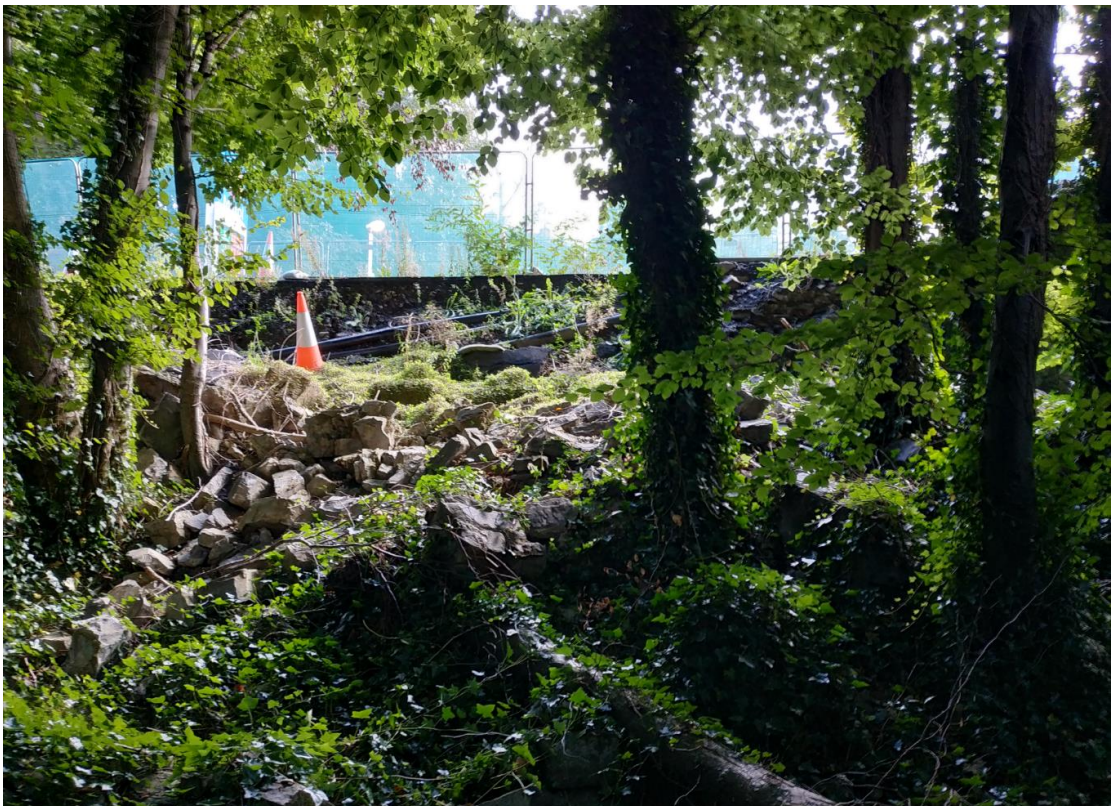
Photograph 5 Looking to the South. Collapsed retaining wall section
