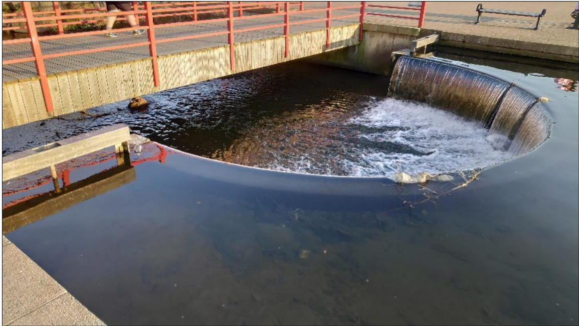
Plate 3.16 The vertical spill-over weir at the outfall of pond P5, March 2021 (the most significant instream barrier to fish passage within the survey area)
