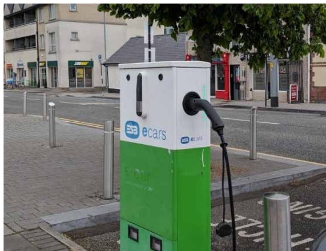
Electric vehicle charging
