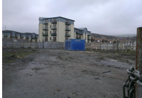
Overgrowth rubble & rubbish cleared from site (port cabins also removed since this picture was taken).
