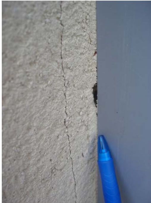
Photograph 24 – Open joints and gaps between rendered reveals and door frame – on rear elevation
