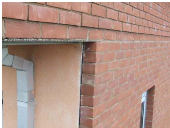
Photograph 14 – Open joints between brickwork and external render finish
