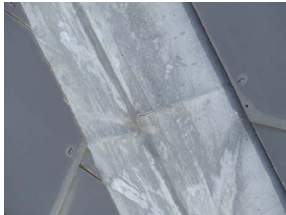
Photograph 5 – Lead valley gutter – splits in the leadwork
