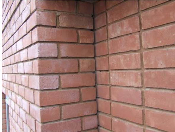
Photograph 12 – Open joint between main external brick wall and recessed brickwork on front elevation
