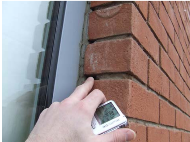
Photograph 18 - Holes and gaps between brick reveal and window frame
