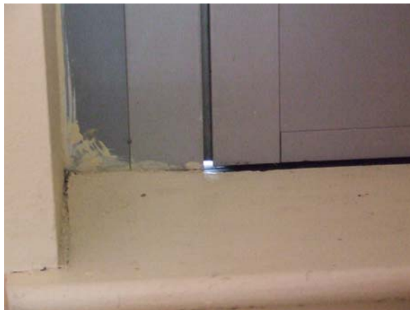
Photograph 21 – Gap and space along bottom of balcony door
