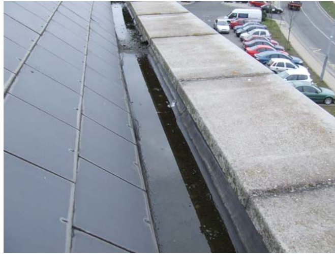
Photograph 4 – Front parapet gutter – ponding and collection of debris and water
