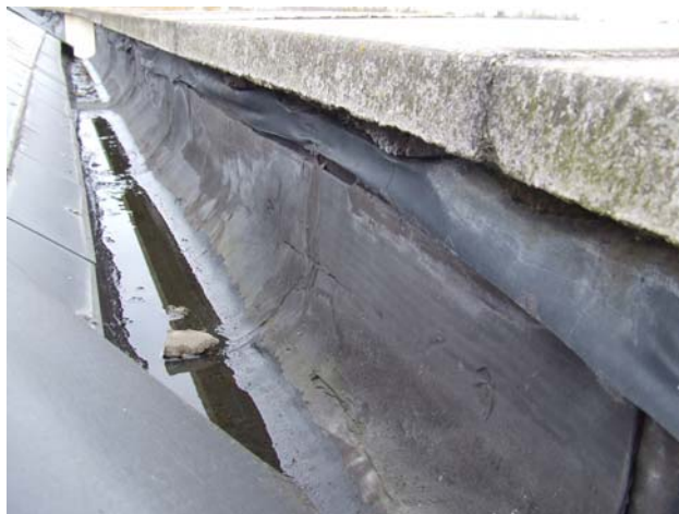
Photograph 3 - Front parapet gutter, open joints and poor detailing
