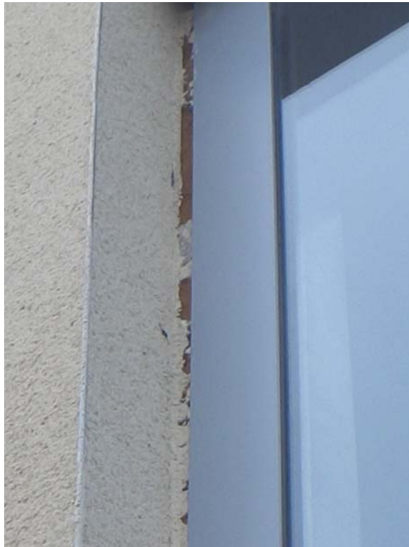
Photograph 25 – Open joints and gaps between rendered reveals and door frame – on rear elevation
