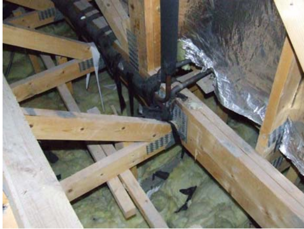
Photograph 33 – Non insulated and exposed copper pipework within main attic areas and spaces
