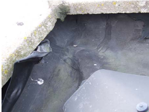
Photograph 6 – Front left hand corner of parapet gutter – poor detailing
