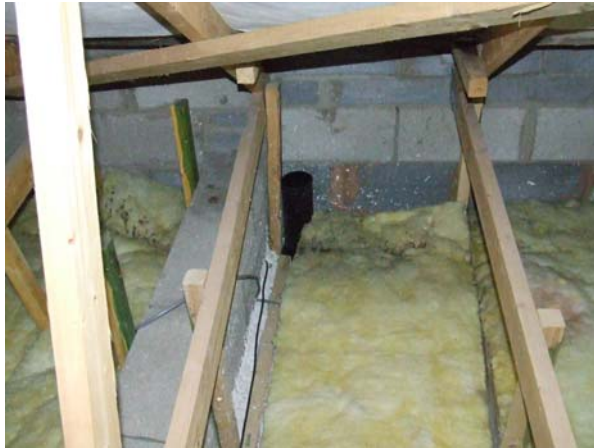
Photograph 30 – Vent pipes terminating within the main attic spaces and voids
