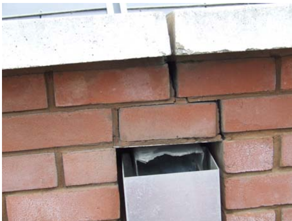
Photograph 11 - Movement and cracking to brickwork above rainwater outlet
