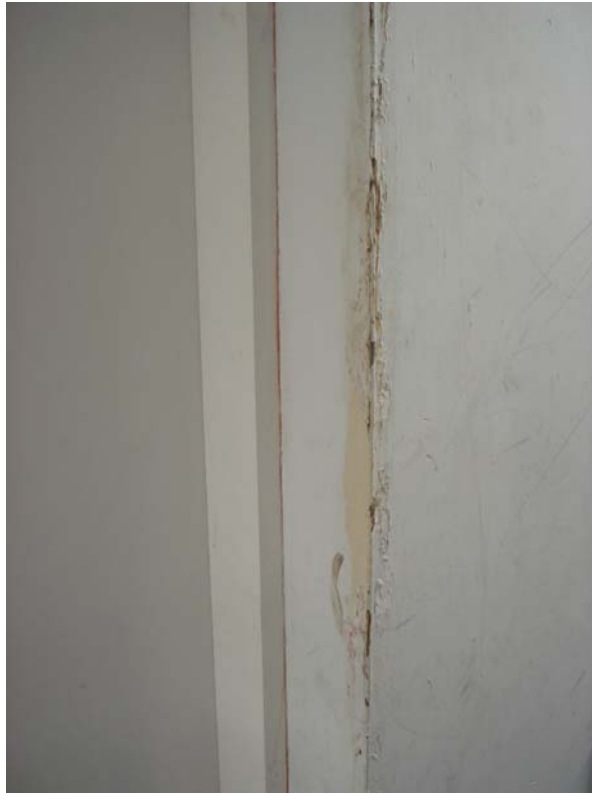
Photograph 28 – Staining and surface corrosion to internal walls adjacent to apartment door
