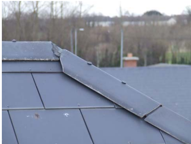
Photograph 2 - Open joints and gaps and mastic material to ridge tiles
