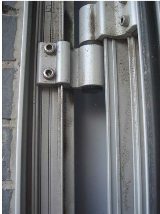
Photograph 20 – Missing rubber and weather seals and strips within the framework and edging of the front entrance doors
