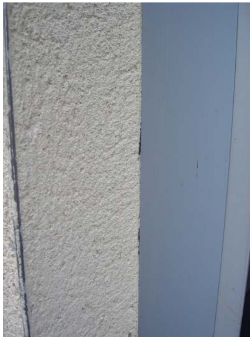
Photograph 23 – Open joints and gaps between rendered reveals and door frame – on rear elevation
