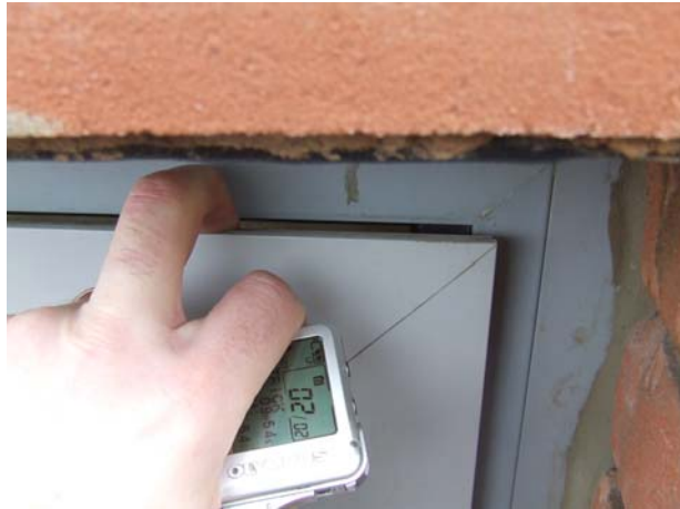
Photograph 15 – Open joint and gap between window light and window frame
