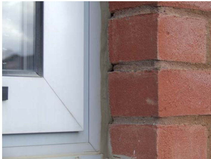
Photograph 16 – Holes and gaps between brick reveal and window frame
