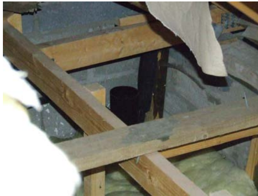
Photograph 29 – Vent pipes terminating within the main attic spaces and voids
