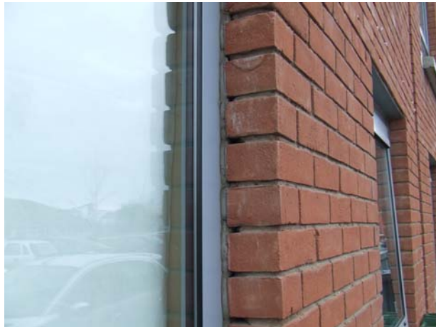
Photograph 13 – Open joints and gaps along junction of window frame and brick reveals
