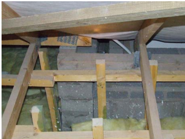
Photograph 32 – Non sealed gaps and spaces and missing fire resistant material along wall between attic and common areas
