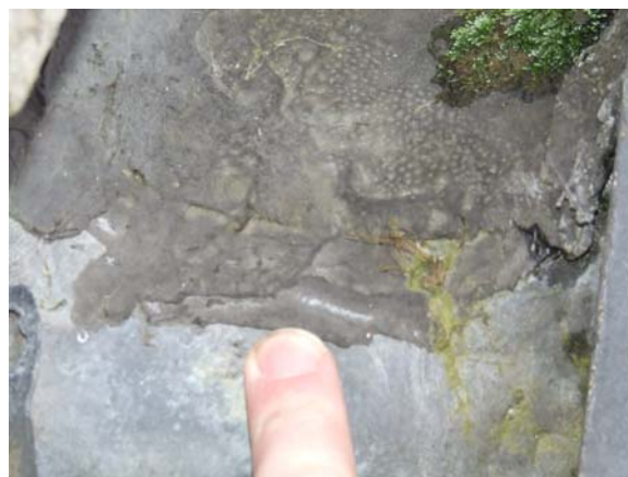
Photograph 8 – Bitumen felt covering to lead valley gutter construction joint – shrunken mastic material
