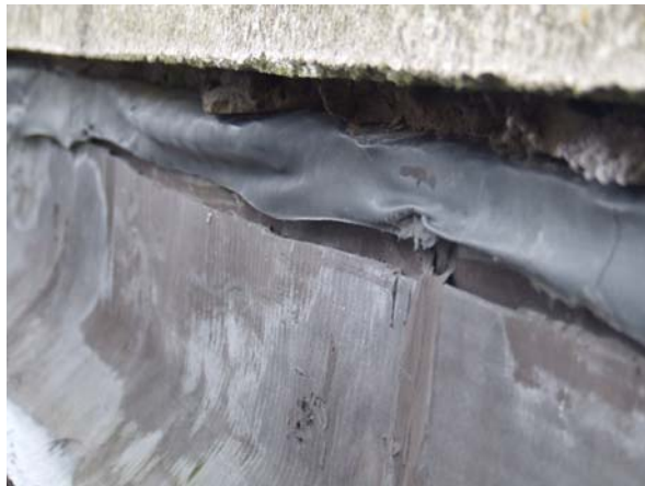
Photograph 7 – Damaged damp proof course material underneath parapet capping and poor detailing
