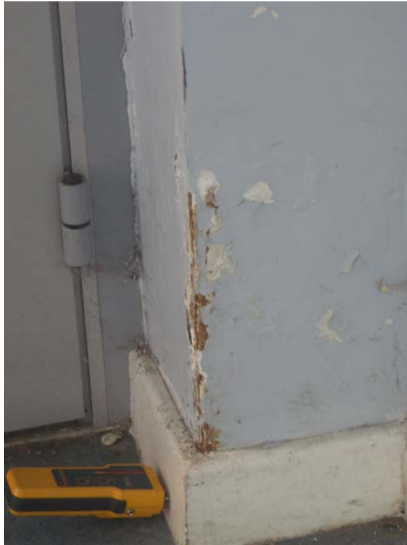
Photograph 26 – Water ingress along bottom corners of rear elevation and rear door
