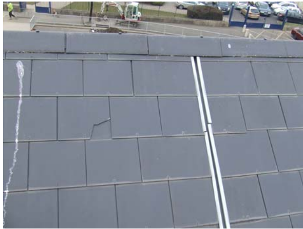
Photograph 1 - Cracked roof tile
