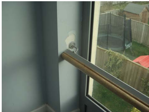
Photograph 27 – Loose and partly detached guard rail to rear window within common areas
