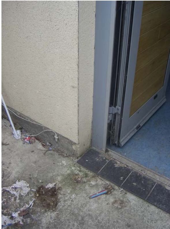
Photograph 22 – Open joints and gaps between rendered reveals and door frame – on rear elevation
