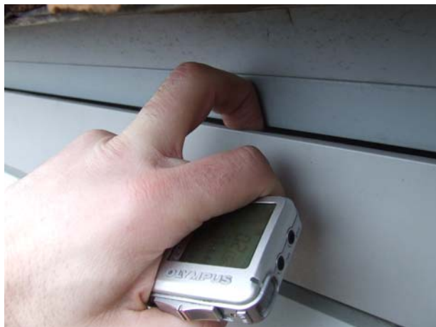
Photograph 17 – Open joint and gap between window light and window frame
