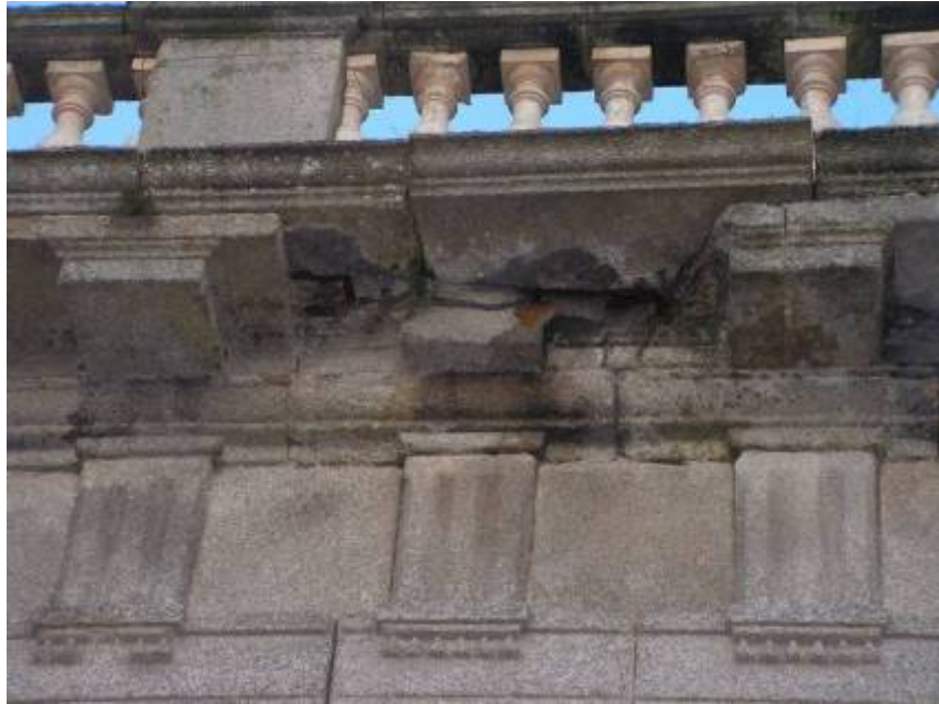
Part of the damaged dentil course of the south-western façade before works began
