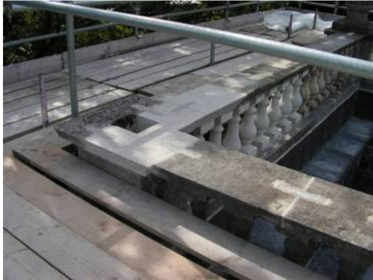
The south-eastern corner of the balustrade during the works. New granite jointed with new stainless steel cramps.
