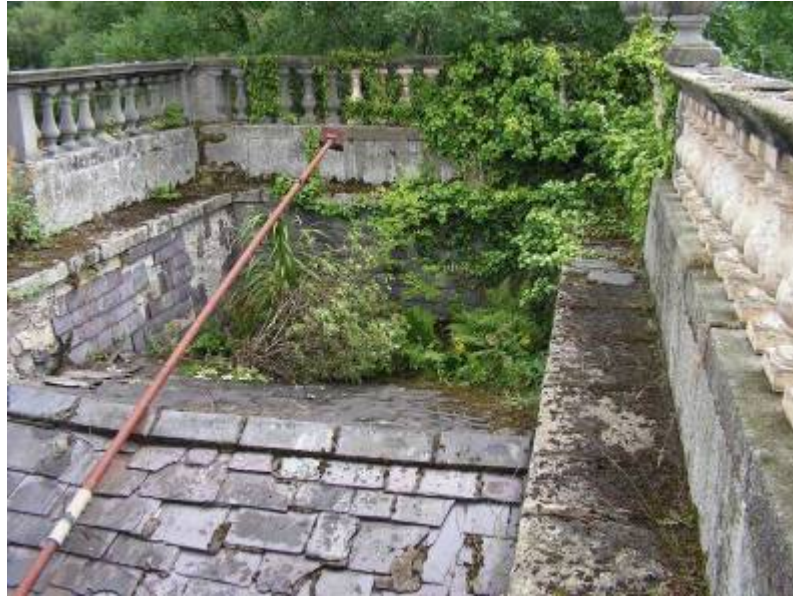
A general view of the roof taken from the north-western corner of the roof before works began
