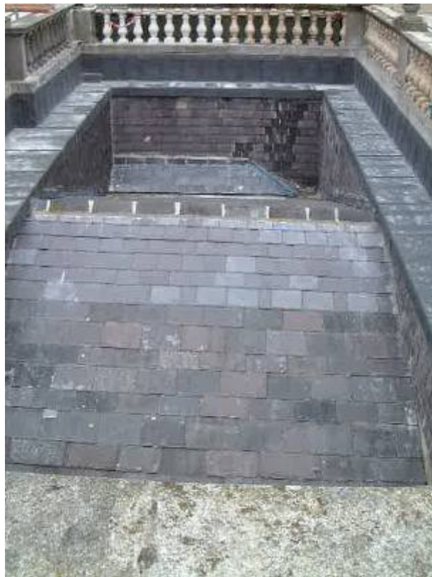
The repaired roof, viewed from the north-west, on completion of the works
